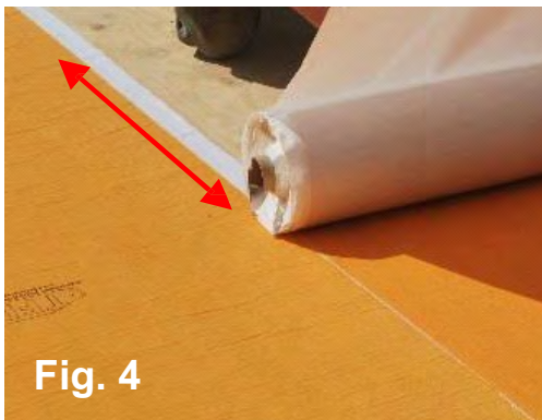
Fig. 4 - Ensure that each new length of mat overlaps on the white strip (shown in Fig. 4) to bond and seal the previous length.
